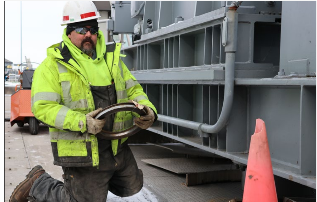
Noah Andow, maintenance and repair, getting a gudgeon pin shims cleaned and ready for installation at Lock and Dam 3, near Red Wing, Minnesota, Feb. 21. USACE St. Paul District photo by Elizabeth Stoeckmann
