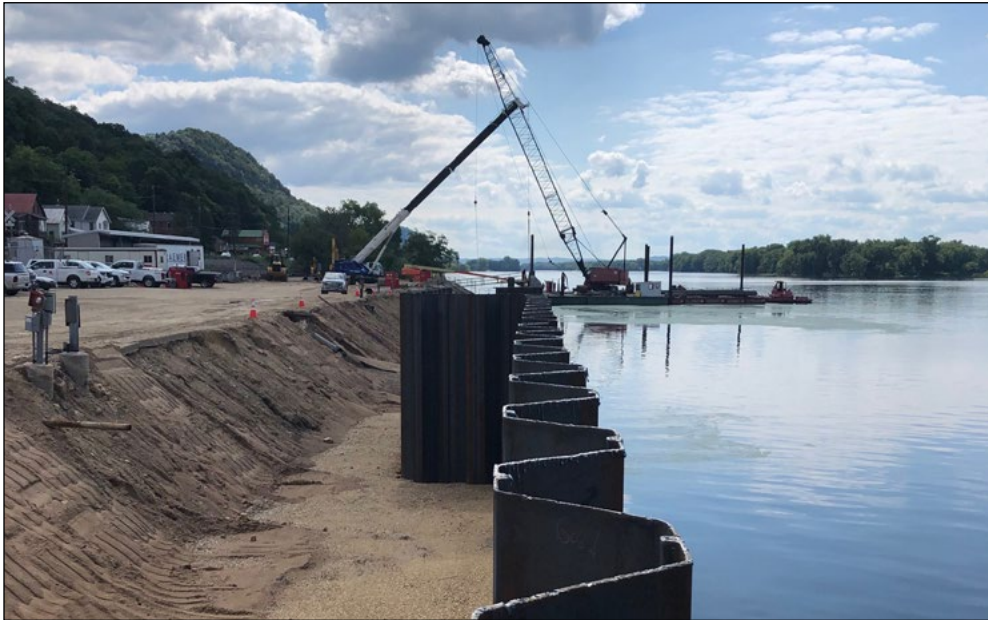
Crews begin work to upgrade the harbor walls at the Fountain City Service Base, in Fountain City, Wisconsin. USACE St. Paul District courtesy photo
